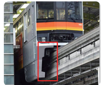
Guide Rails of Monorail Tracks
