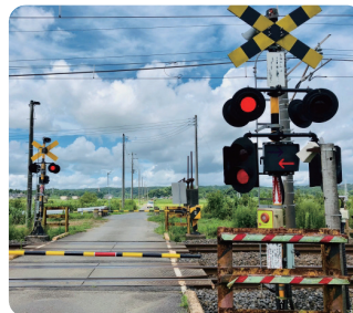
Sensors for Railways
